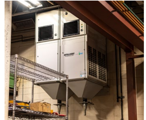
IVEC GVSC with mobile housekeeper system
