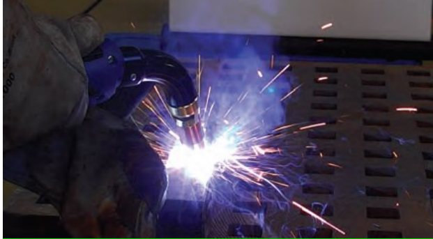
Fume Extraction Source Capture Suction is OFF
